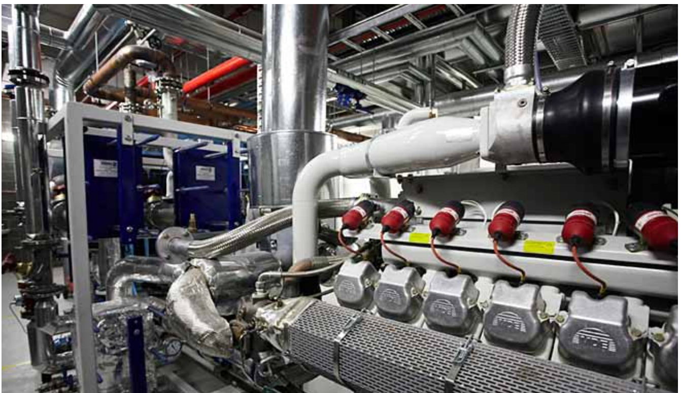
image courtesy of Cogent Energy
