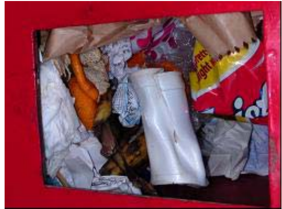
Photograph 19 Litter Contained Inside Fire Hydrant
