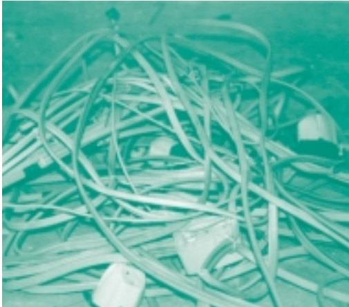
Stack of electrical and data cable.
