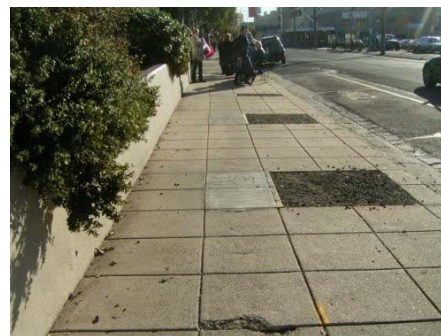
Photo 21 Plants removed, damaged paving
